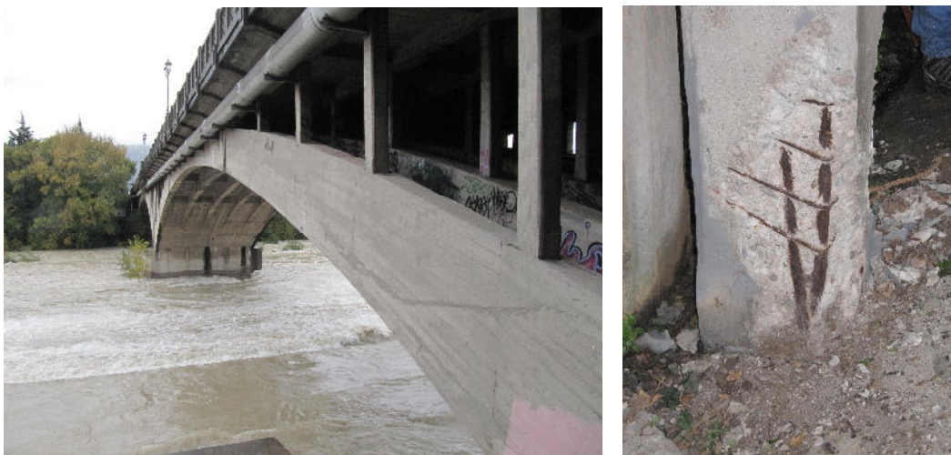
Figure 5: Downstream arches seen from left-hand side abutment; substantial concrete loss of mass
